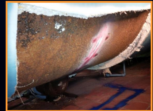
Crack in ESP Chiller
