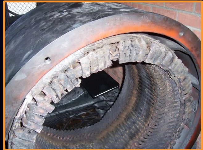
Aging Elevator Motors
