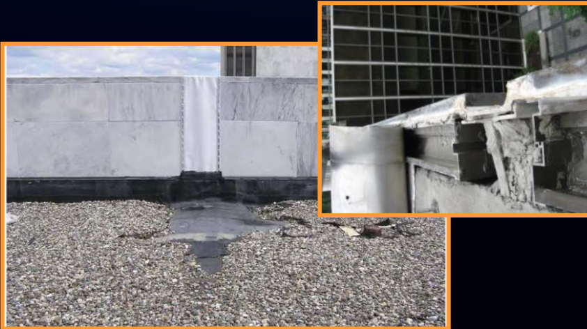
Holes in Roof Membranes
